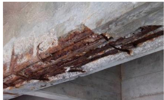
Fig. 1. Damage to concrete members due to corrosion of reinforcement
