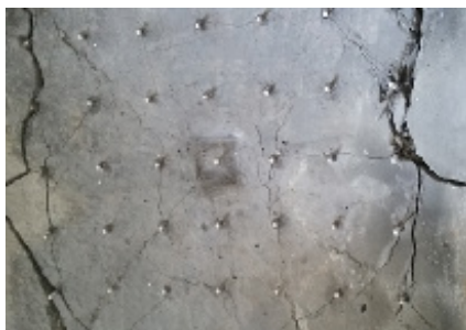
(d) removal of upper plate and observation of cracks on the concrete surface
