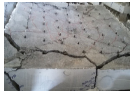
(e) development of internal cracks of the concrete to the external surface of slab
