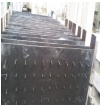
(c) installing the moulds and setting up the slabs vertically for concreting
