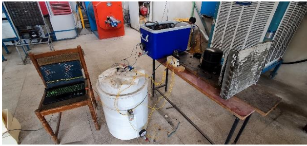
Fig. 1. Constructed direct-expansion solar heat pump system.
